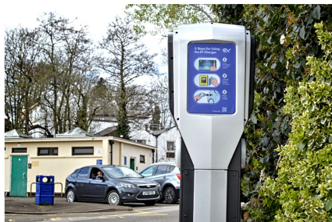
New EV charging point in Abergavenny
